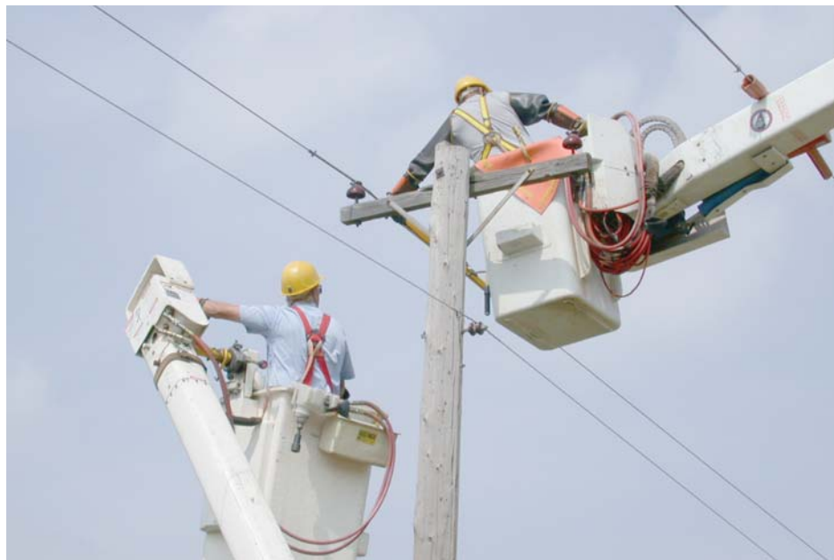
Clark Electric linemen worked on upgrading a three-phase line this past summer.
