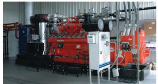
The Generator —After the gas goes to the top of the pit, it is then pumped to this generator to produce electricity. It can generate up to 600 kw of electricity.
